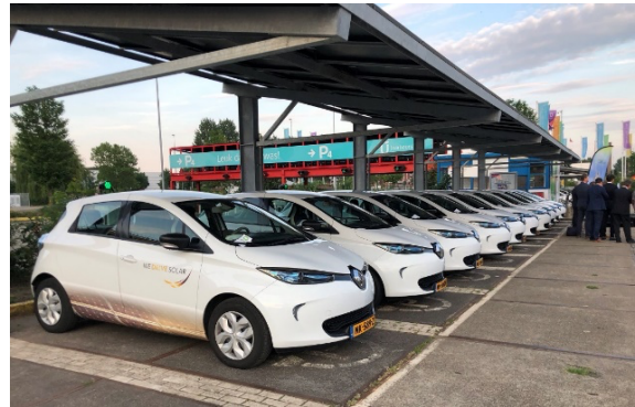
Figure 2. Bi-directional (AC V2G) charging points and roof with solar panels in the testing ground Utrecht Station area, The Netherlands
